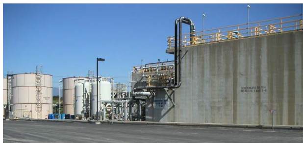
Figure 1 – Leachate Treatment Plant (LTP)
