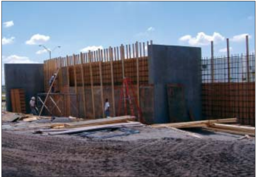
The Mid County Station was constructed with three drop-off bays that utilize three 100 yard transfer trailers. The modified West County Station will incorporate this new design to improve capacity.
